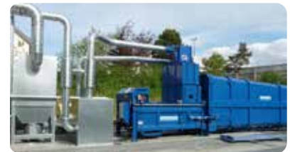
STP for a printing company
