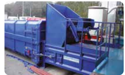
STP with bin lifter at a loading dock
